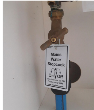
Photo: water mains stop tap under kitchen sink
