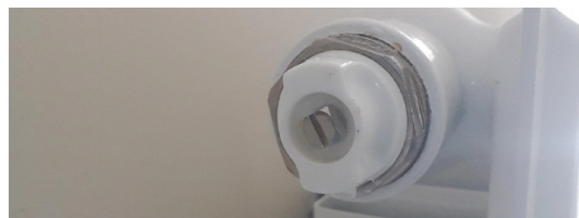
Photo: radiator bleed valve)
